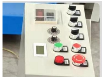
Control the electrical components of the whole machine operation
